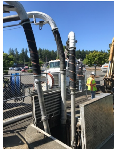
Vacuum trucks keep wet well levels in control during valve vault upgrade.
