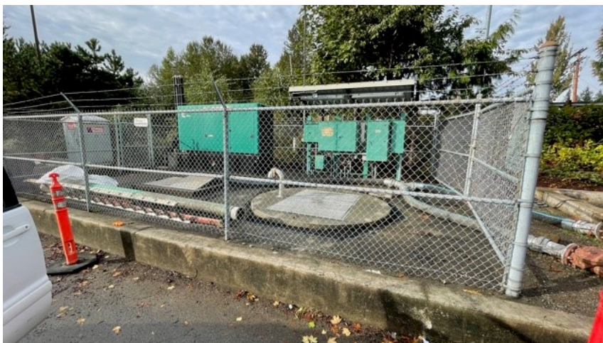
Liftstation #18 with upgrades install including new generator.
