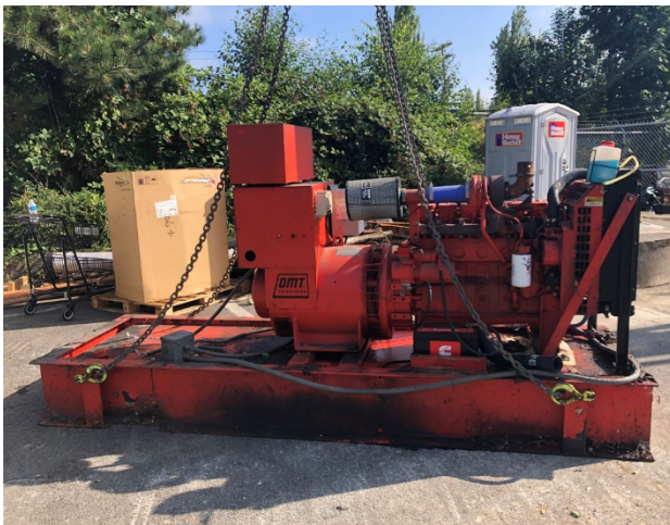
Original diesel backup generator.
